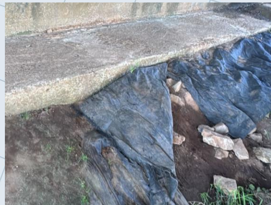
Exposed abutment footing with dislodged erosion protection
