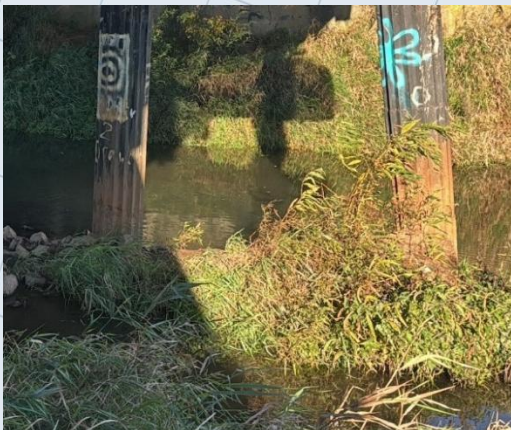
Steel-encased concrete piles showing corrosion
